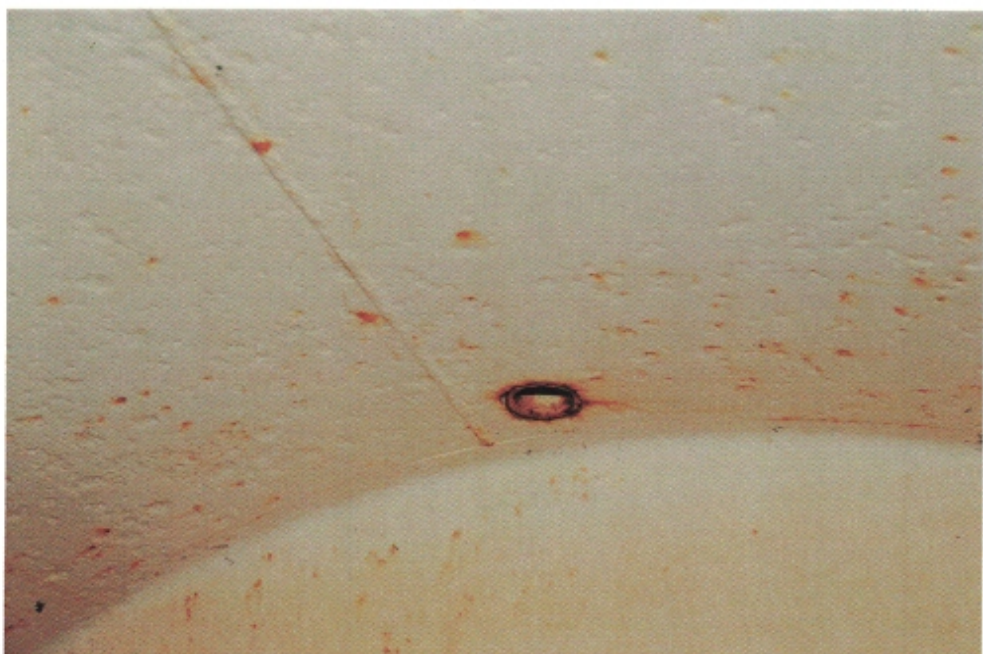
I-12 View of the upper portion of the reservoir, illustrating moderate corrosion at the circumference of a capped penetration and minor corrosion on the adjacent surfaces.
