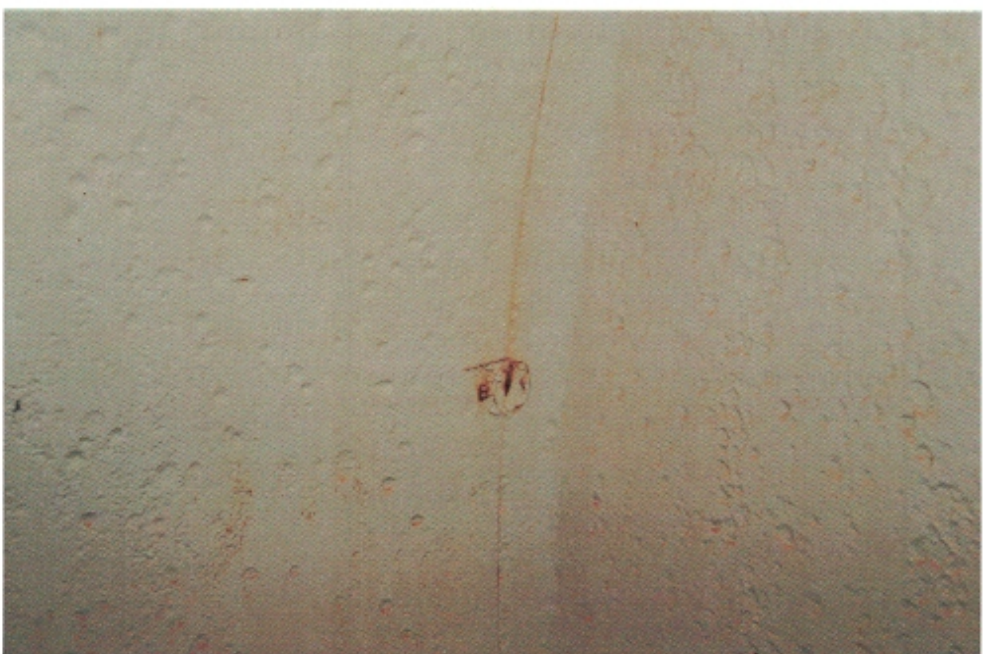
I-13 View of the shell where it meets the dished head, illustrating a defect at the weld and minor corrosion on the adjacent surfaces.
