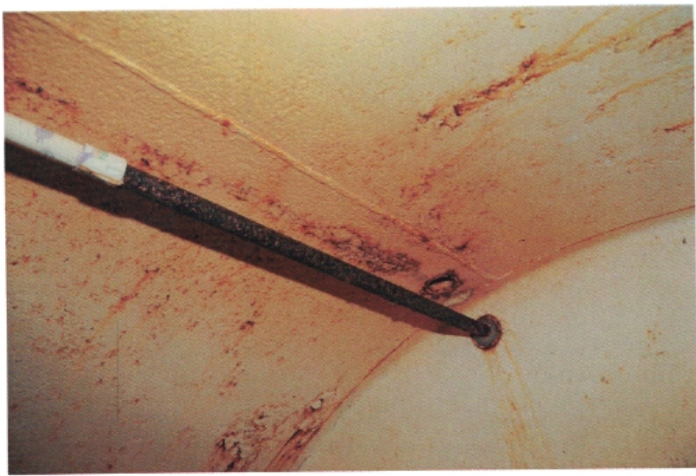
I-8 View of the inlet pipe where it enters the reservoir, illustrating severe corrosion of the carbon steel portion of the pipe.
