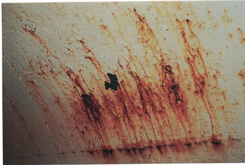
I-6 Same as Photos I-4 and I-5, except in a different location. Note area where the coating is starting to delaminate from the substrate.
